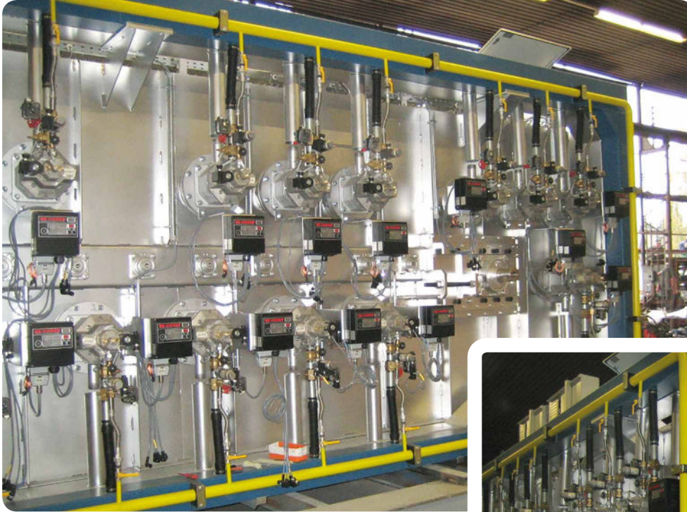
Hardening Furnace w/ Gas Radiant Tube Heating and Energy Efficient Recuperative Burners
